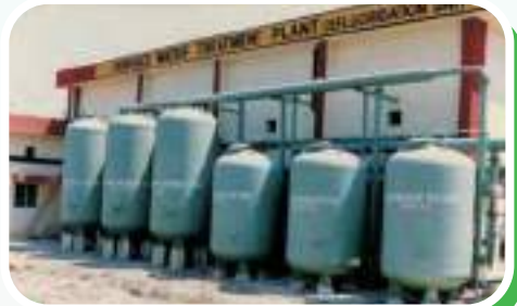
Fluoride removal plant for community drinking water systems
