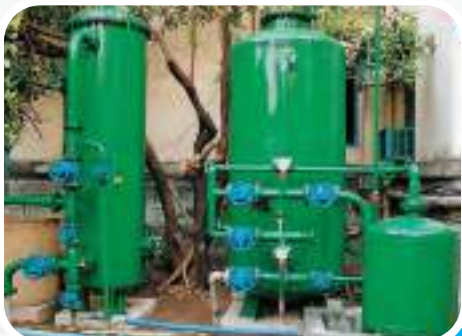
Iron removal & softening system for housing society
