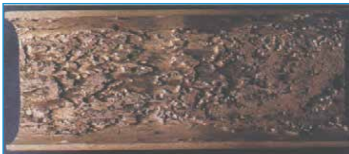
Fig 10.7 - Photograph of boiler tubes with deposits
