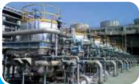
Demineralisation plant for a refinery project
