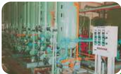
Softening plant at a sugar mill
