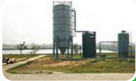
Continuous sand filter for surface water treatment
