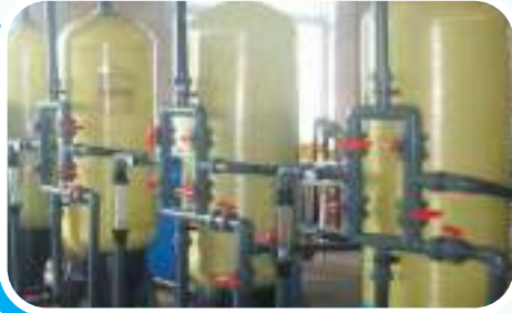
Arsenic removal plant for ground water treatment
