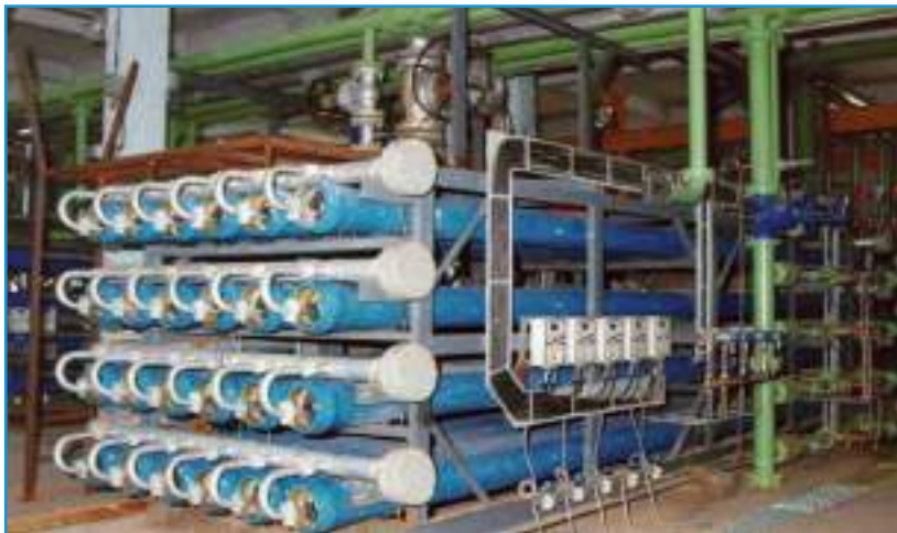
Fig 11.7 - Photograph of fully assembled RO skid
